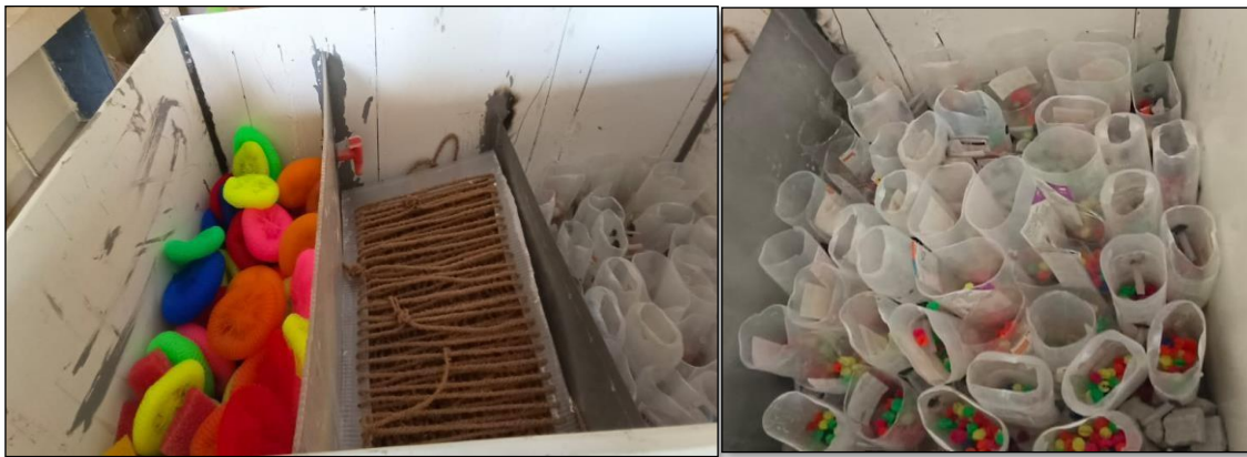
:Reactor Tank A
