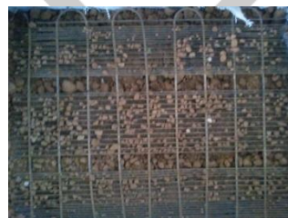
[Fig.10 Loop of copper pipes]
