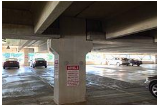
Fig1.2: Precast parking structure showing an interior column, girders, and double-tee structural floors. The two gray circles are covers to close the lifting anchor holes.
