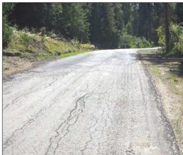
Fig.1 Current Pavement Issue.
