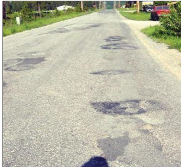
Fig.2 Extra patching is more expensive than FDR.
