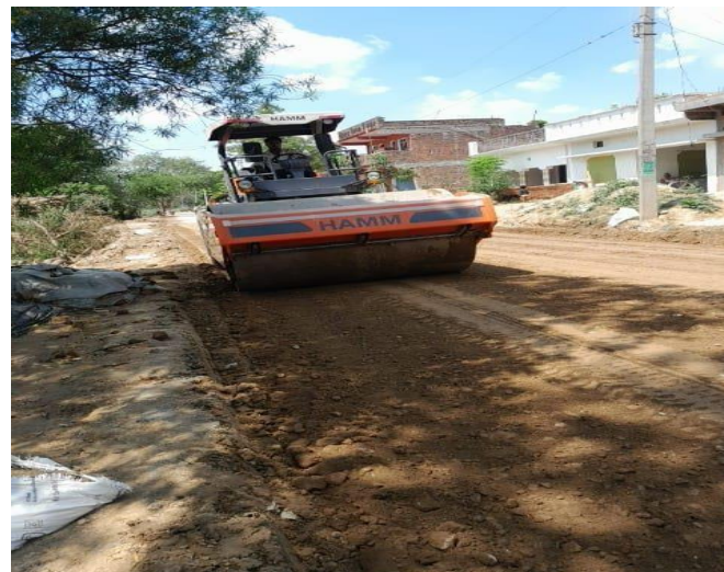
Fig.7 Equipment and on site testing.
