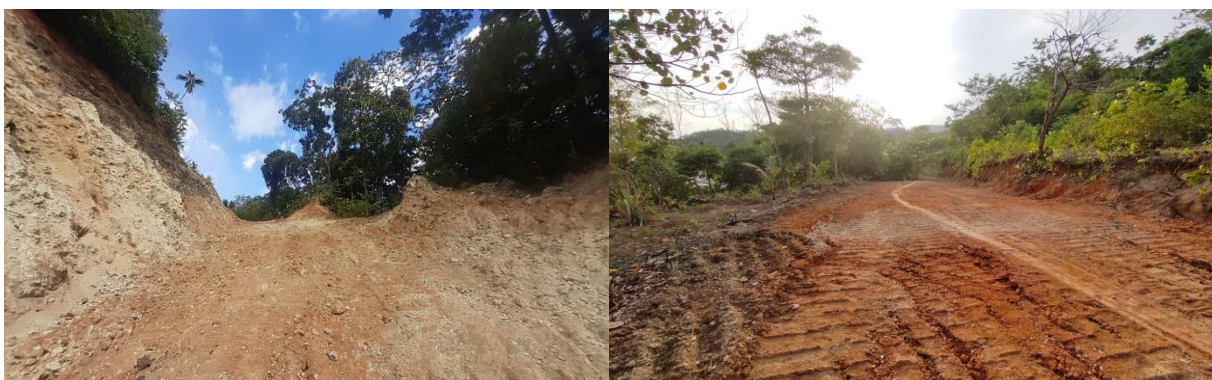
Figure 3 Condition of the Wassu-Oma road at STA 3+325 – 3+350
